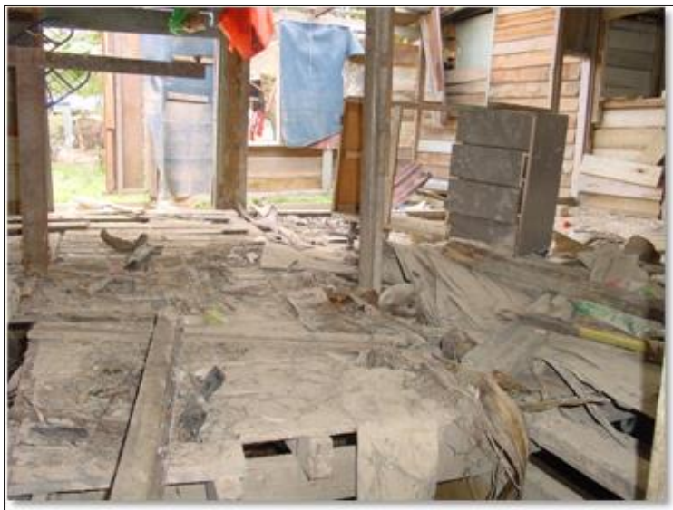
Figure 2: A flood-damaged house whose owner has moved out of the study area. (Source: Field survey)
